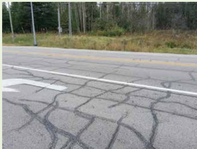
Six-year-old highway with premature cracks in Coldwater, Ontario.
